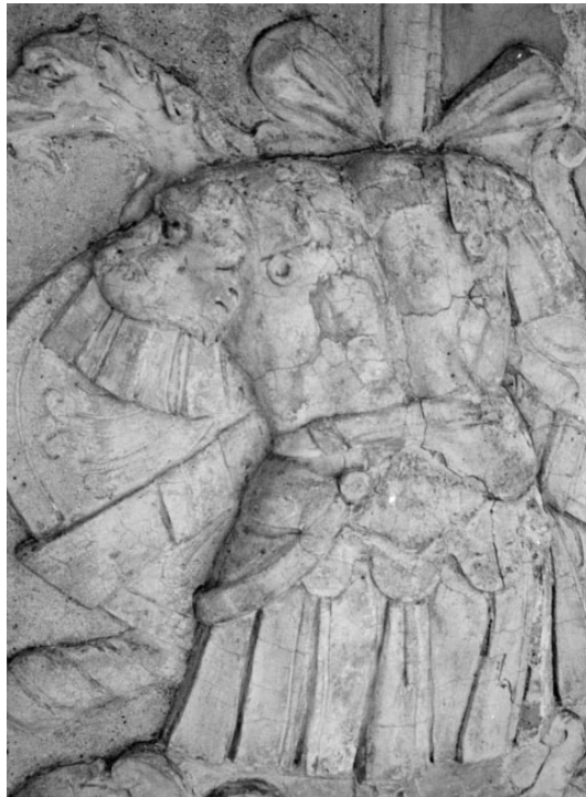
8. Detail of the stucco decoration on the elevation of palazzo Nicolosio Lomellino in Strada Nuova in Genoa, during the restoration.
