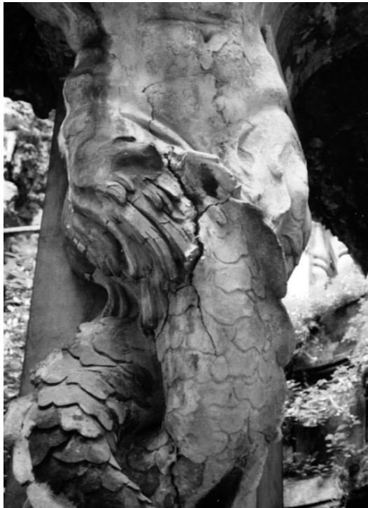
9-10. Detail of the nymphaeum of palazzo Nicolosio Lomellino in Genoa, before restoration
