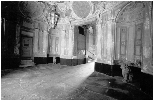
2-3. Detail of the atrium of palazzo Nicolosio Lomellino in Genoa, before restoration.
